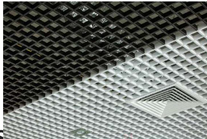
Chequered open grid false ceiling
